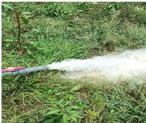
Fig. 2: Wastewater effluent discharge point
